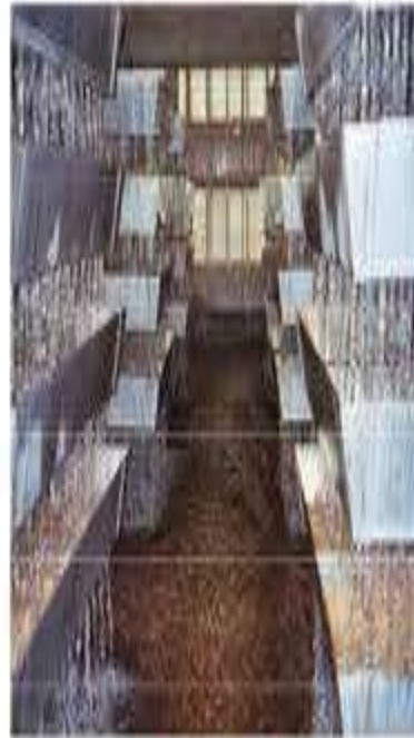
Multi Tray Aerators
